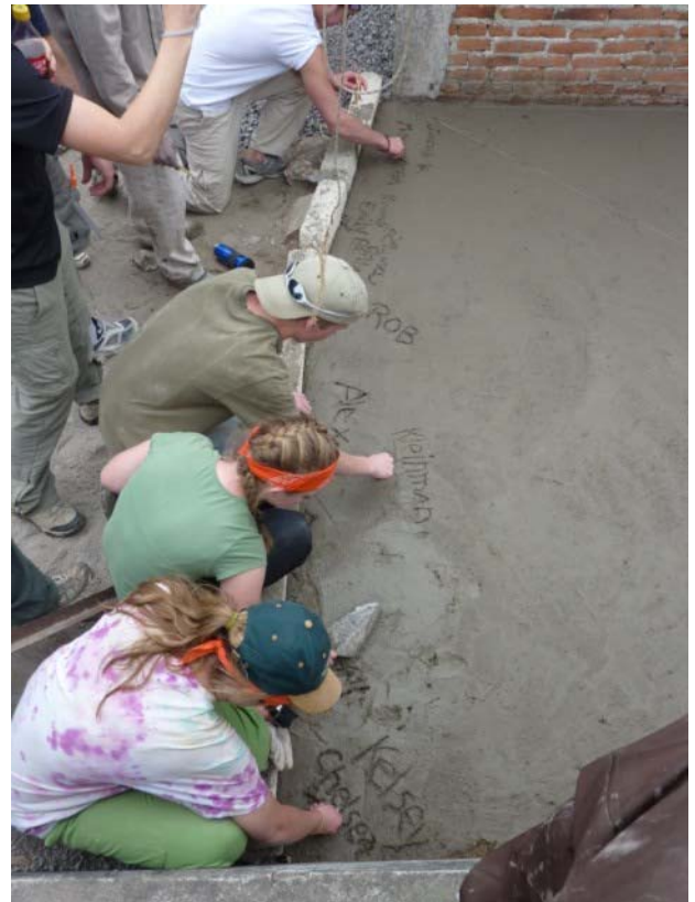
The Mexican family for whom this concrete floor was laid by AHS students was so grateful that they asked the students to please sign their names in the wet concrete so that the family would always be reminded of the gift.
