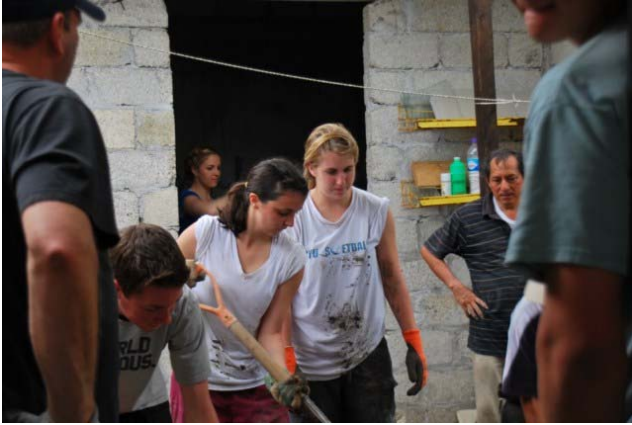
AHS Students prepare to lay concrete on a previously dirt floor in a home in Mexico. They hardly noticed the squelching heat!
